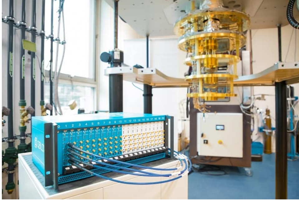
Figure 5.1: Qblox control electronics connected to a quantum computer. Source: Qblox.
